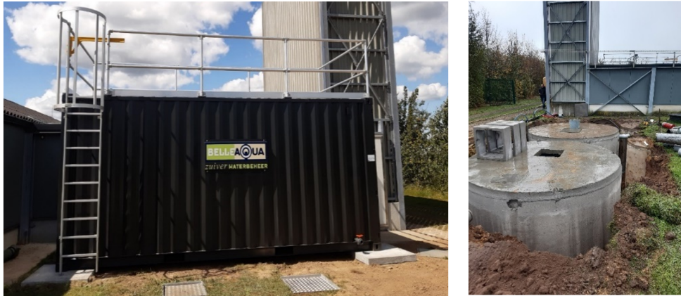
Photo 4: Container setup for cleaning water treatment with underground storage
