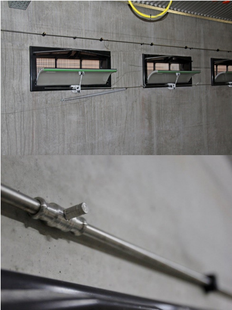
Spray cooling with spray nozzles at the level of the air inlet valves (Photo Experimental Poultry Centre)
